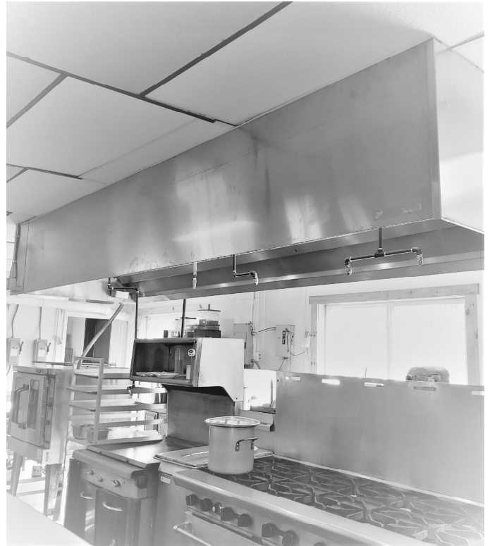
Our New Ventilation Hood/ANSUL Unit
